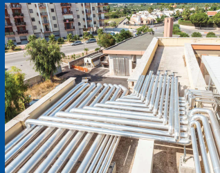
High Pressure Water Supply
