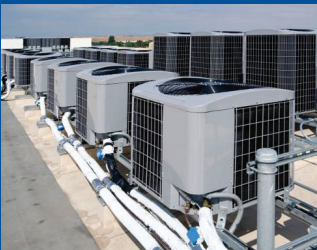
Air Condition or Cooling System
